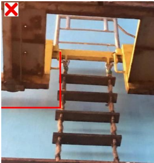
Figure 2 - Non-Compliant Trap Door Arrangement
